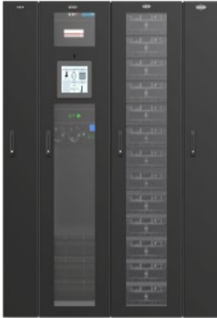
CRAC + Power cabinet + IT cabinet + CRAC
