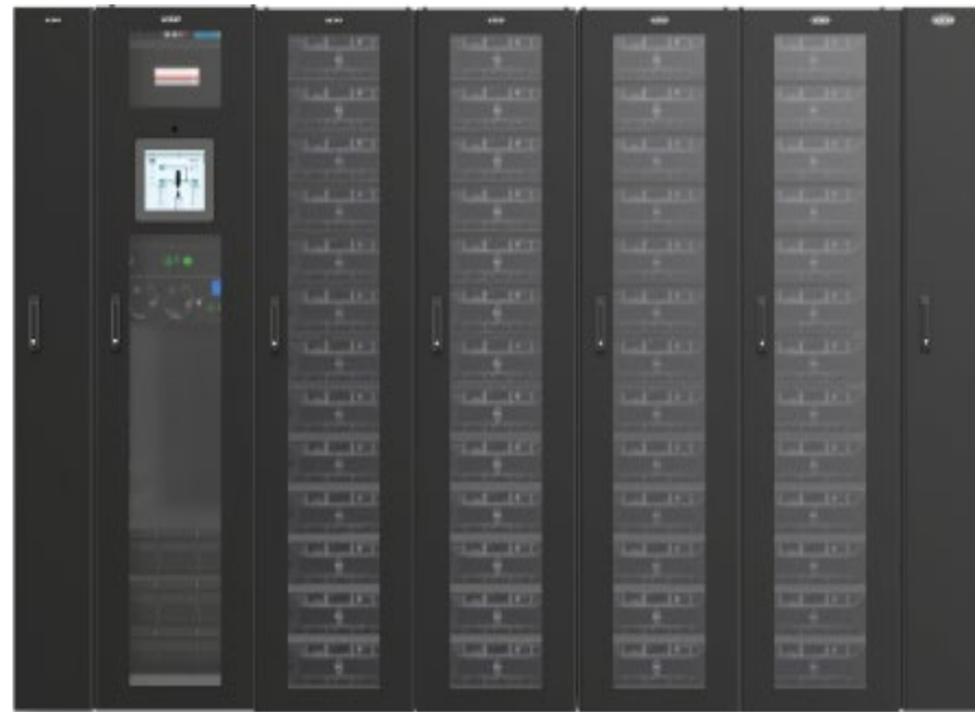
CRAC + Power cabinet + IT cabinet + IT cabinet + IT cabinet + IT cabinet + CRAC
