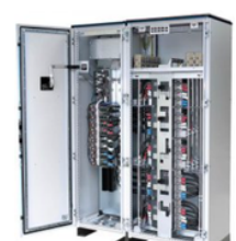
Static Transfer Switch
