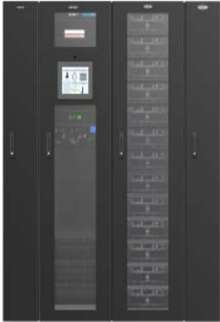
CRAC + Power cabinet + IT cabinet + CRAC
