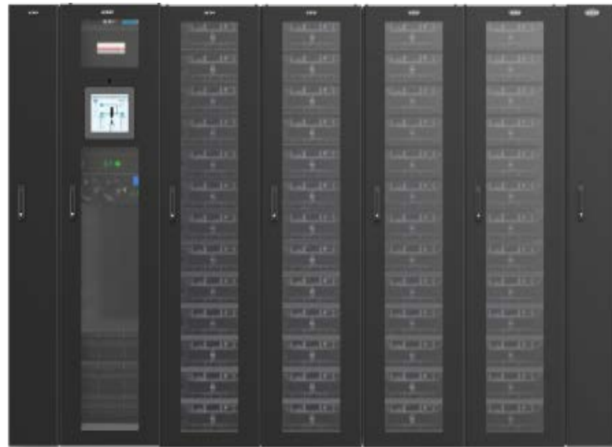
CRAC + Power cabinet + IT cabinet + IT cabinet + IT cabinet + IT cabinet + CRAC
