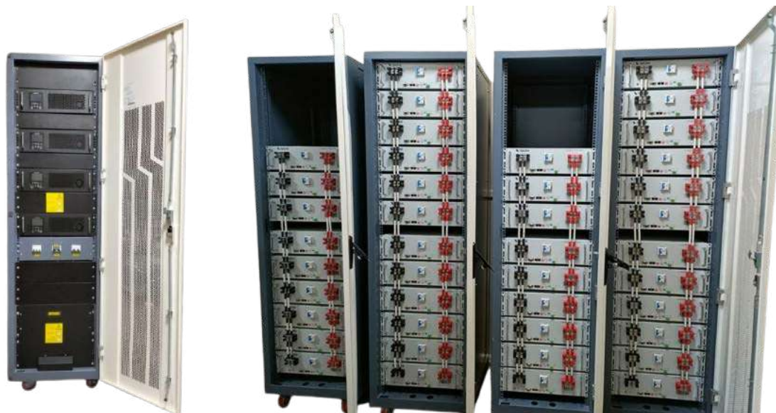
Battery Racks for Extended Back-up time
