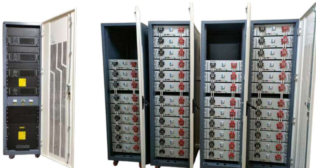
Battery Racks for Extended Back-up time
